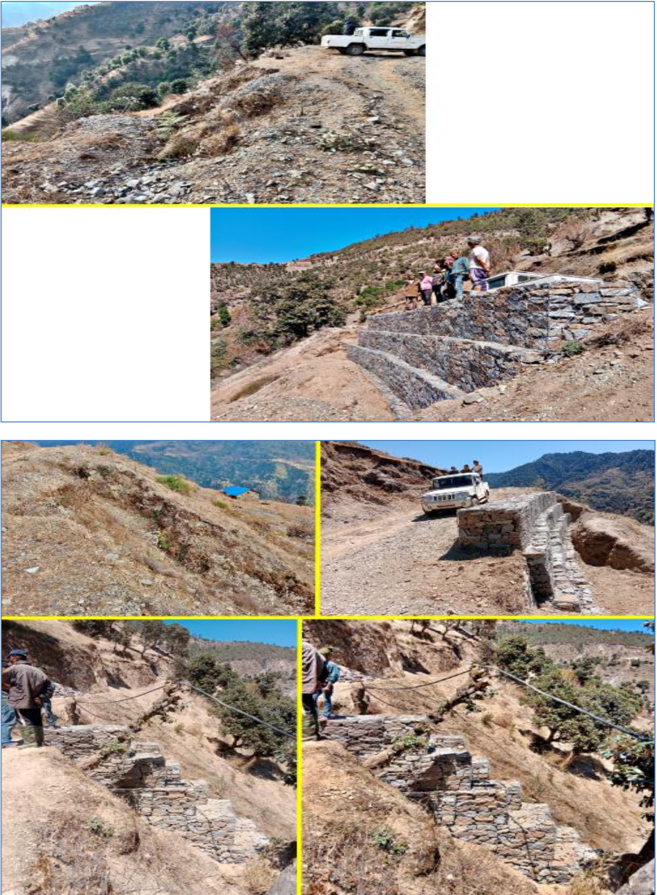
Figure 416: Gunam Gully & Landslide Treatment
