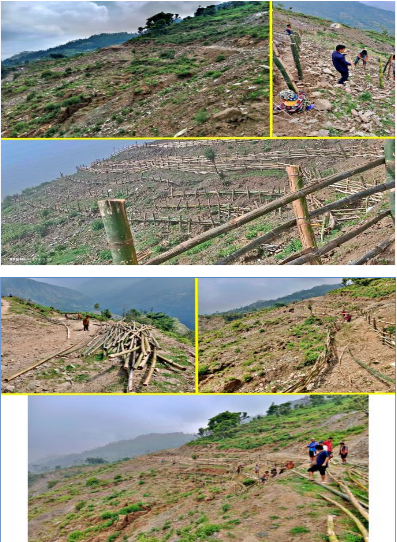
Figure 20: Fagam Landslide Treatment
