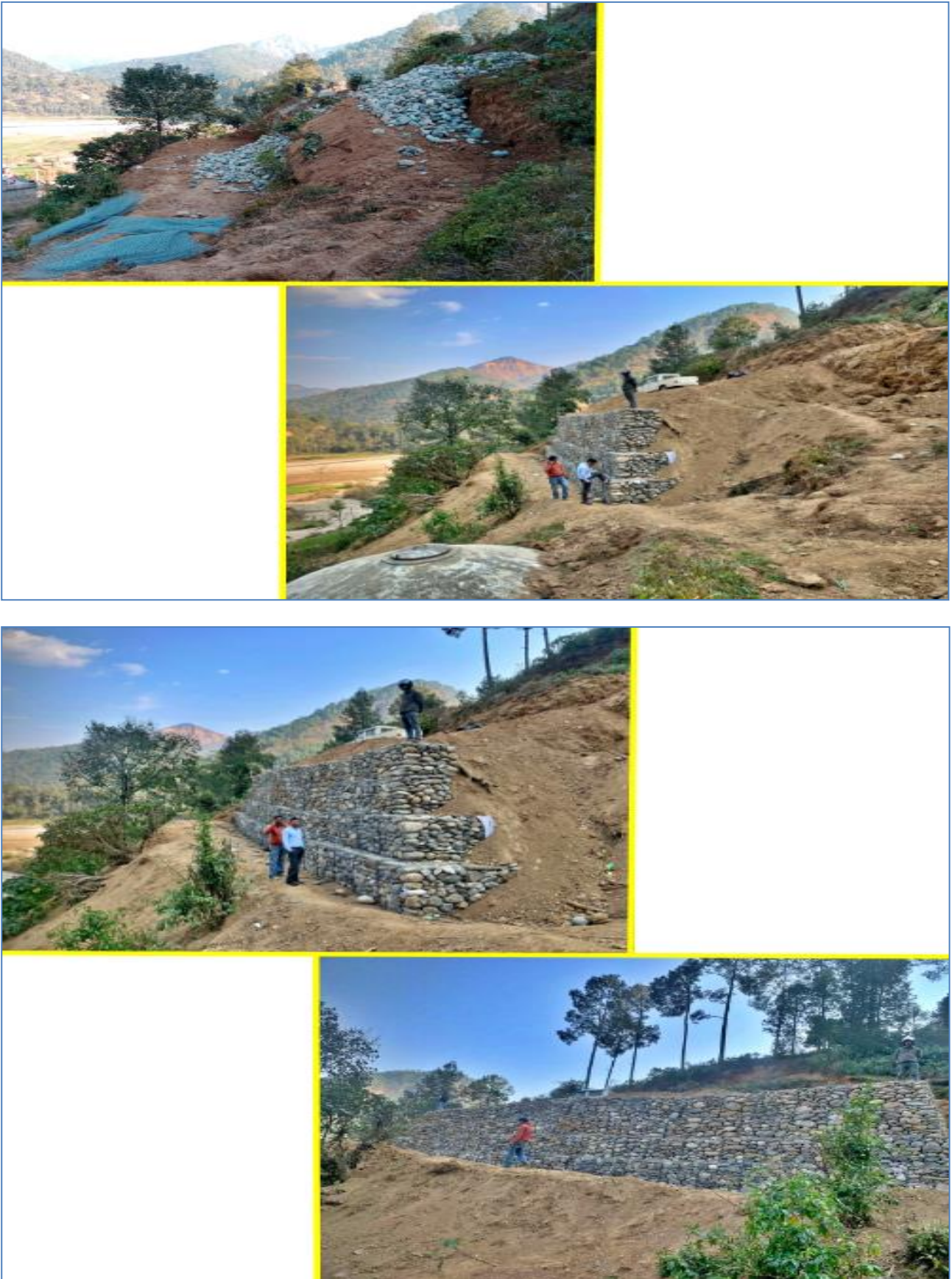
Figure 55: Kaprakhola Landslide Treatment
