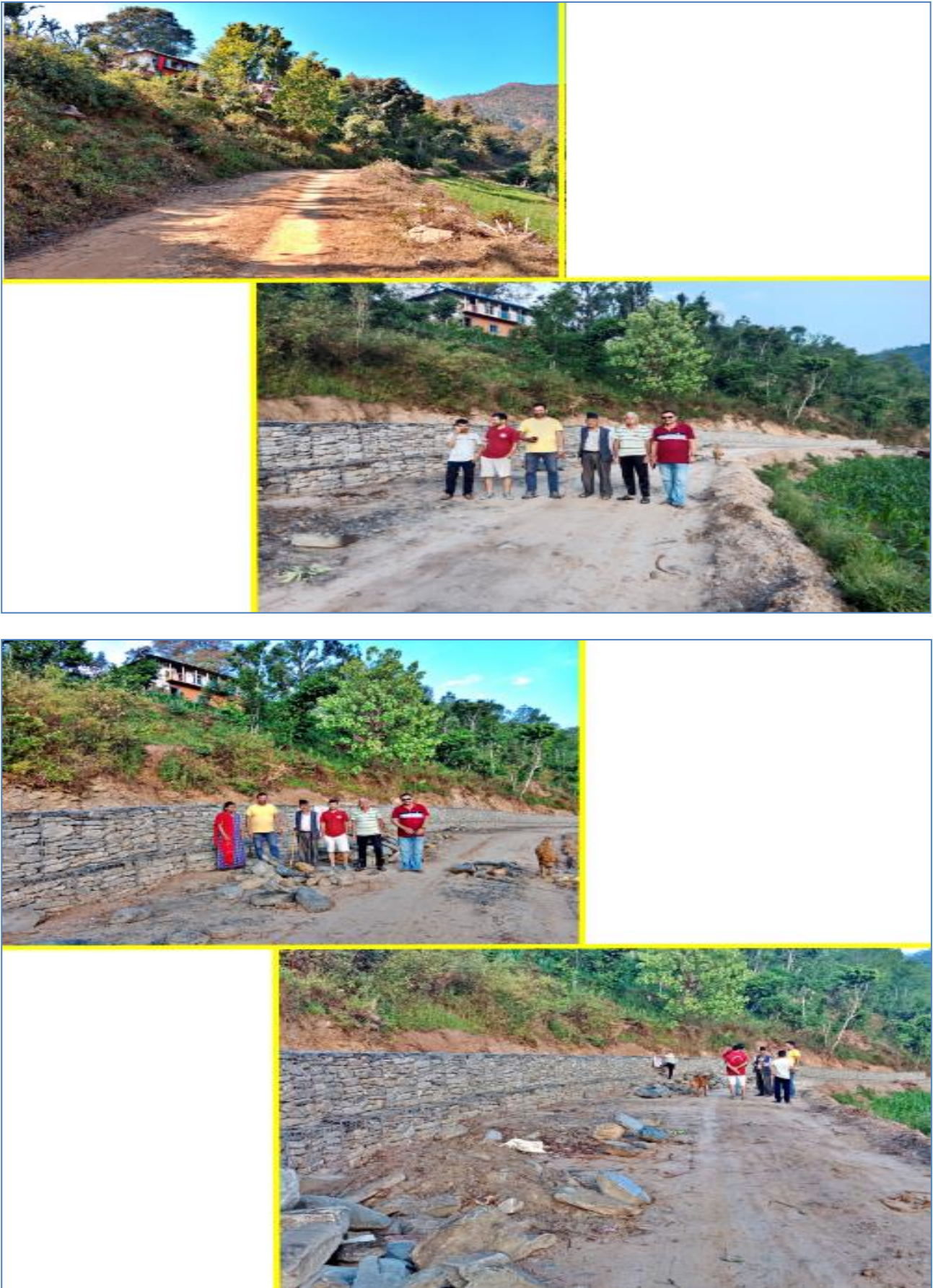
Figure 51: Koladada Landslide Treatment
