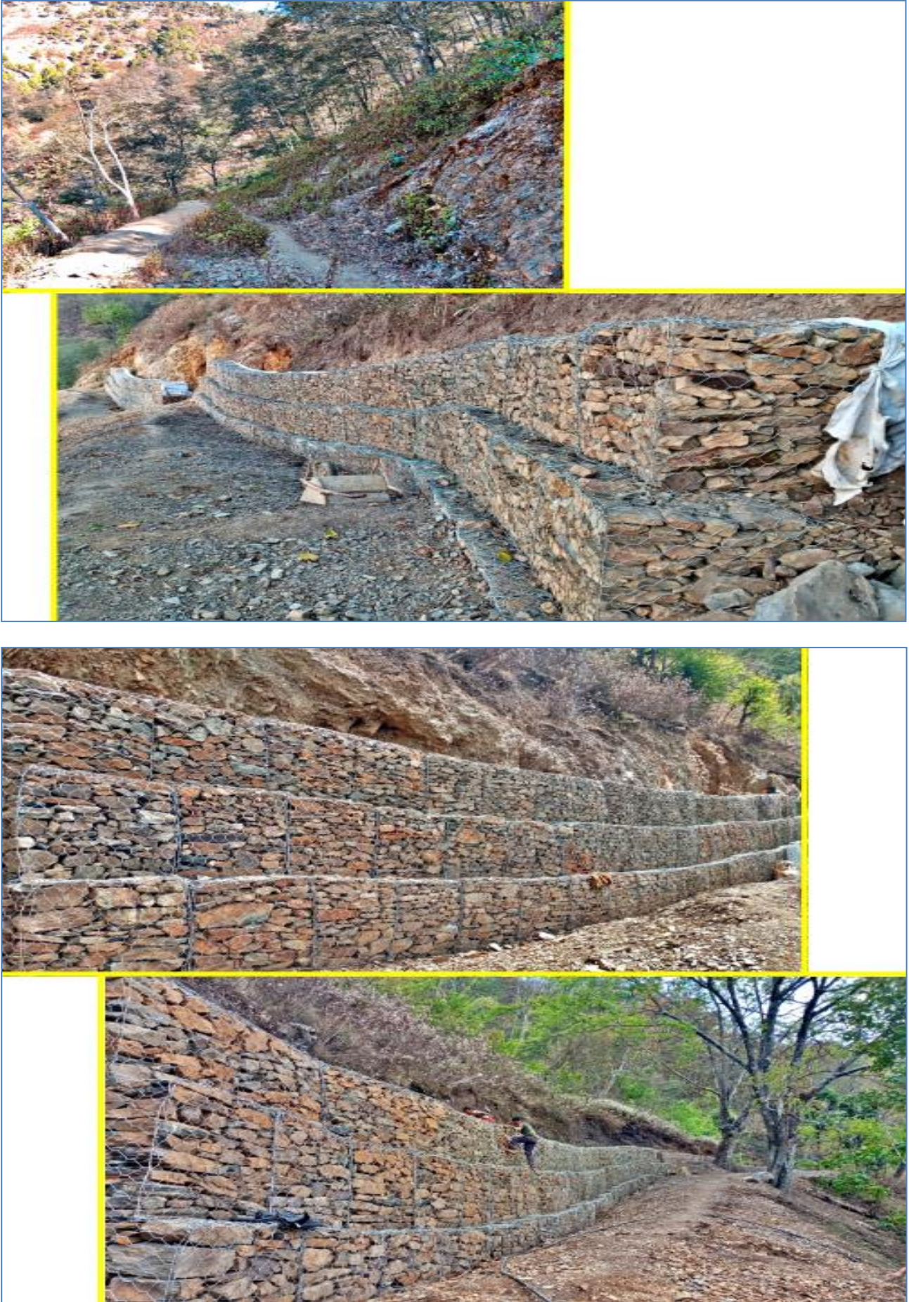
Figure 57: Ghatchaur Landslide Treatment
