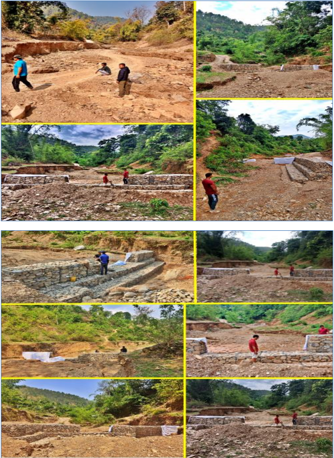
Figure 53: Barkhola Gully Treatment
